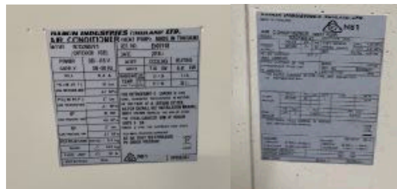
Fig B3 - Installed air conditioning for commercial tenancy
